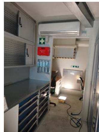
AC Unit above opening to office section
