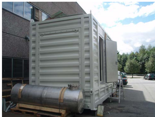
Generator exhaust silencer waiting to be installed. Installation hatch for generator on end wall.
