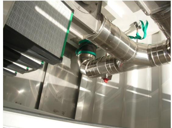
Inside the HVAC module on the roof
