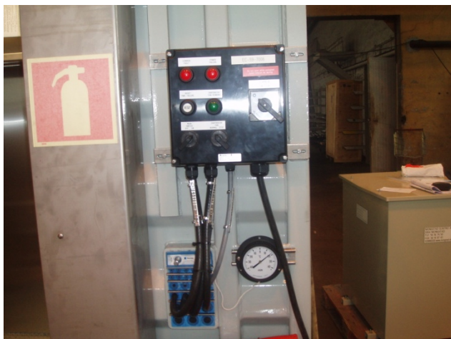
Panel for AC Split Unit
