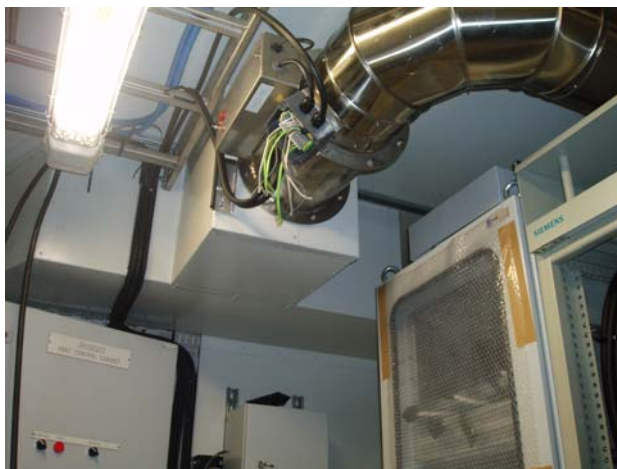
Air inlet with A60 fire damper.
