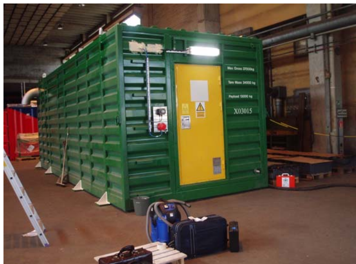
Completed UPS container, ready for delivery.
