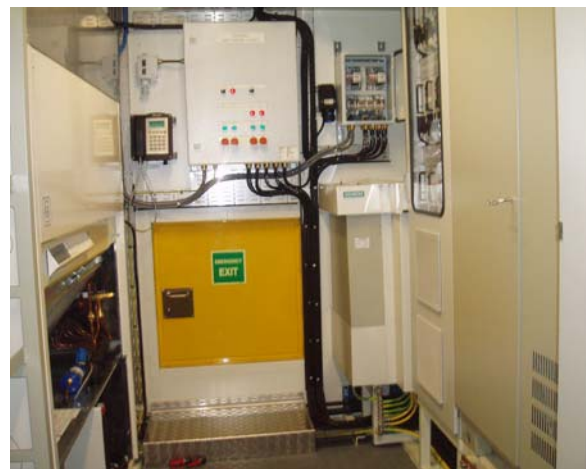
Inside the container, emergency escape panel, mounted under HVAC control panel.
