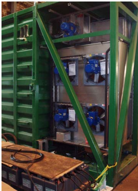
Air cooled condensers mounted outside the container
