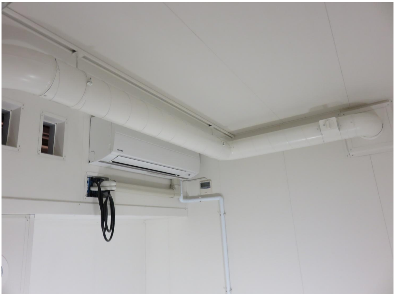
Internal AC unit and ventilation ducting in the container
