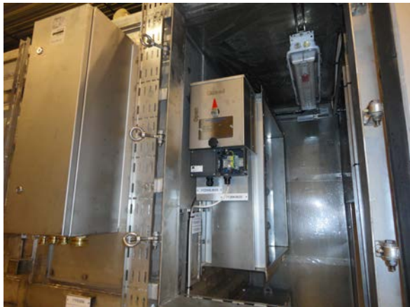
Inlet plenum with lighting and shut off dampers
