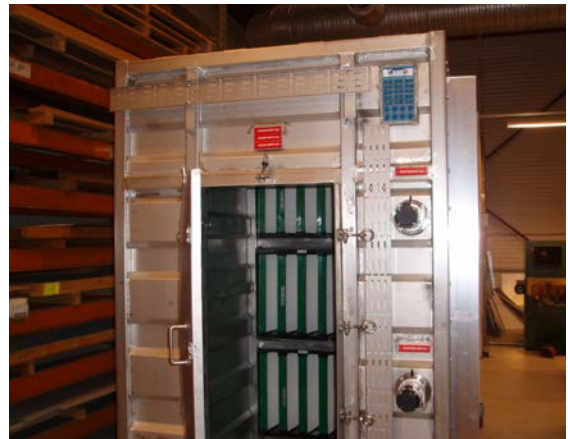
Main inlet section, showing access to filters
