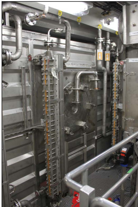
Second floor, weak acid tank
