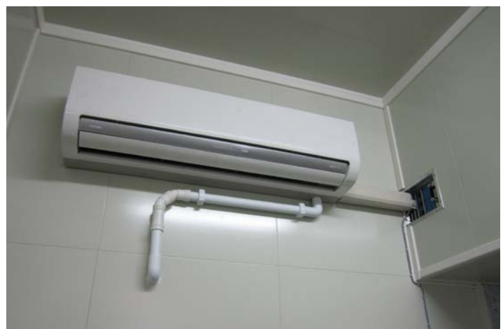
Split AC unit mounted on internal respatex panels, MCT in side wall
