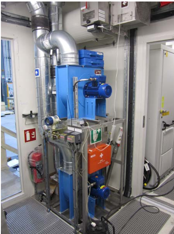
2 x 100% ventilation system and internal ductwork
