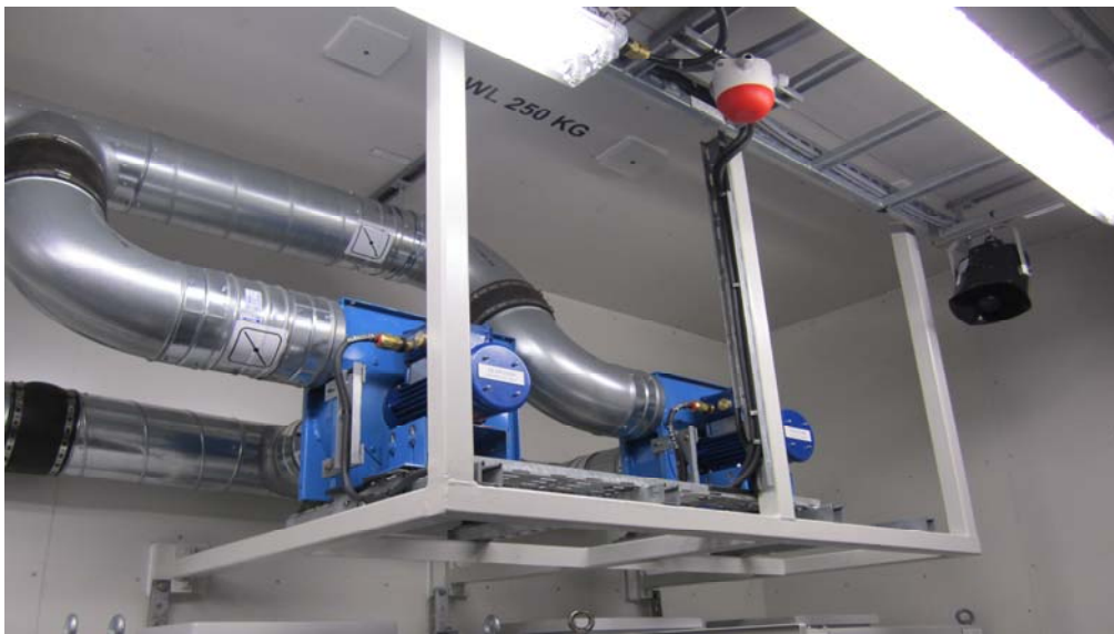
Fresh air Ventilation system
