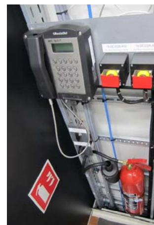
Telecom + emergency stops
