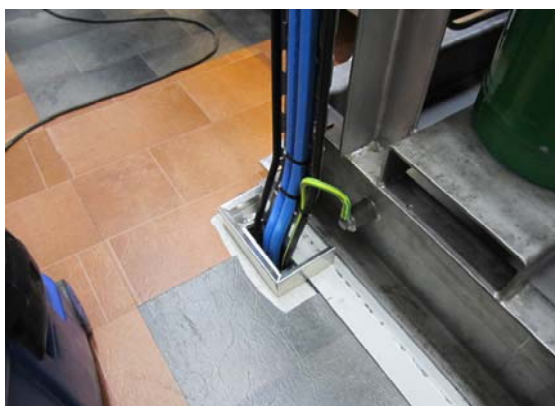
Cables penetrating the suspended floor
