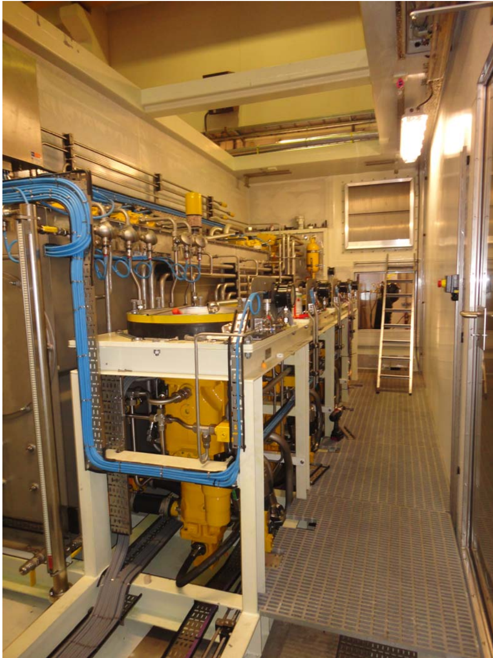
The HPU installed in the container
