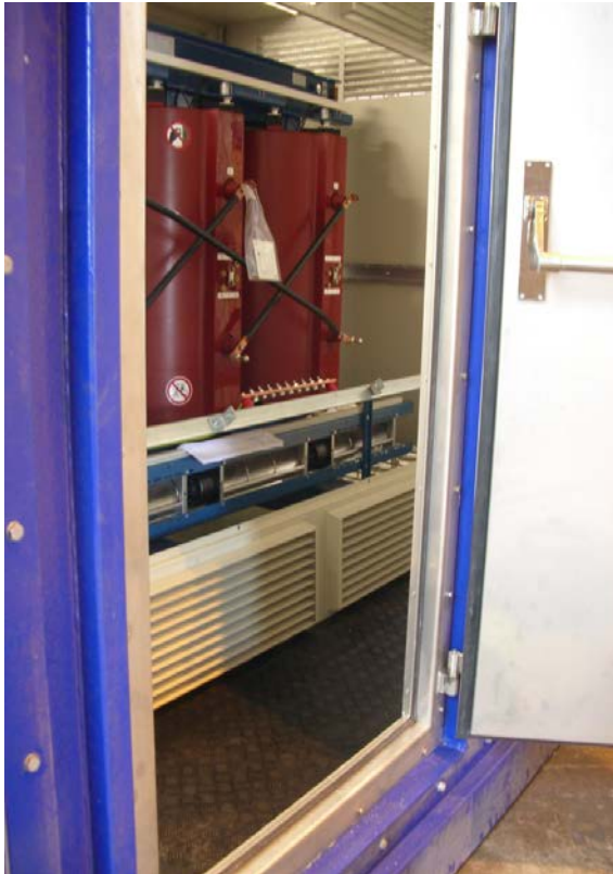
View through the container door into the trafo room
