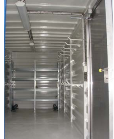
Normal and emergency lighting
