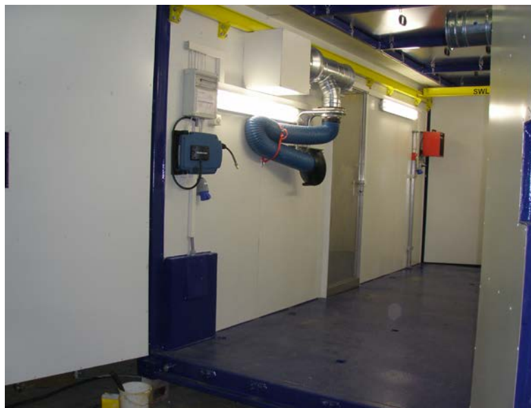
Internal layout, welding extract mounted on the wall on the left.
