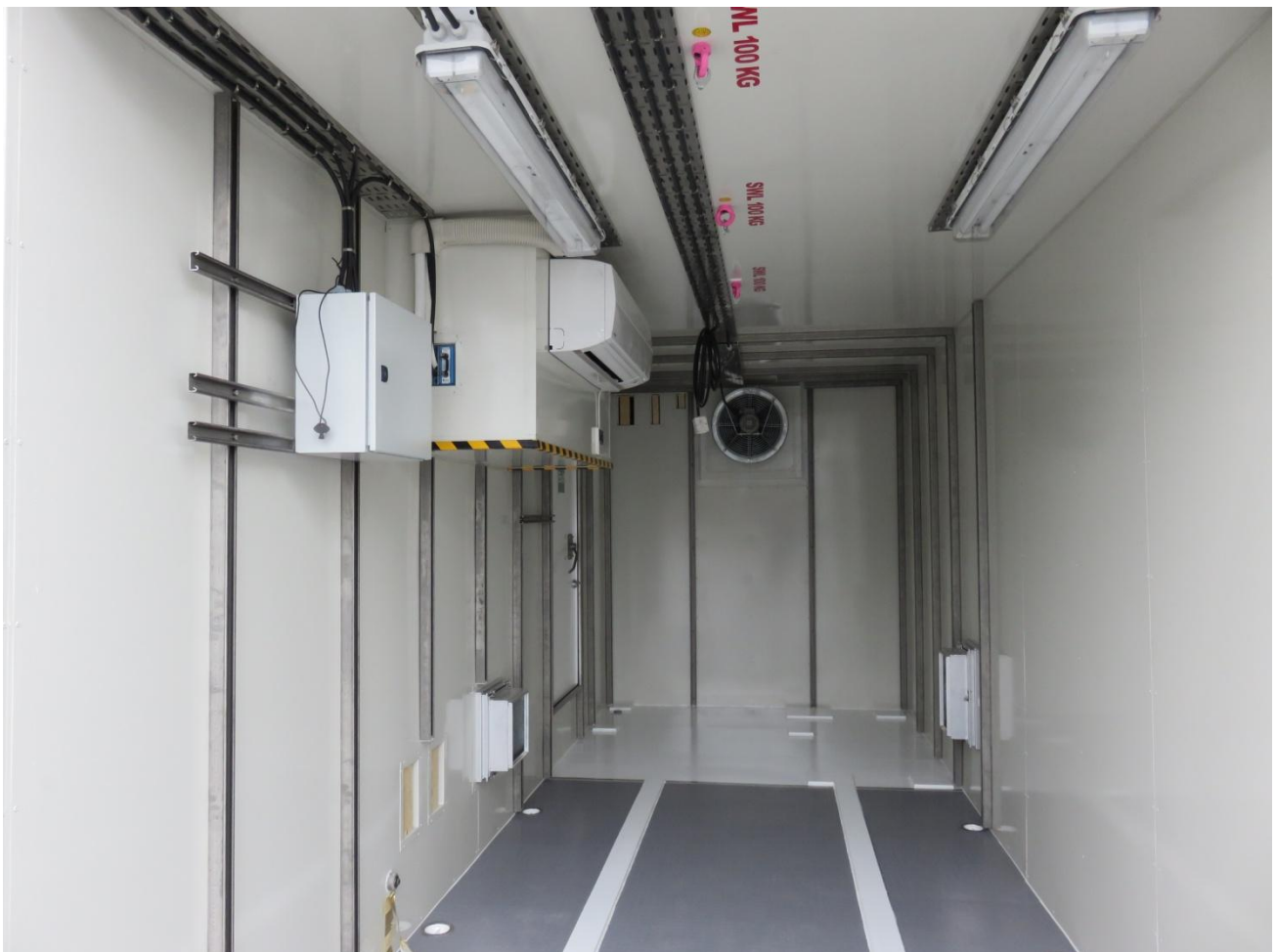
Internal view of the container, showing the installed equipment
