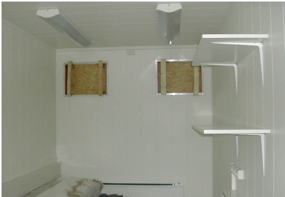
Internal layout, showing openings for A/C units, lighting and shelving
