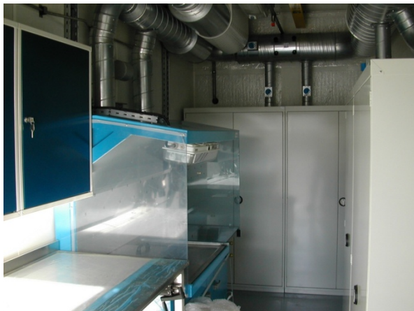
Paint spray cabinet + ventilation system
