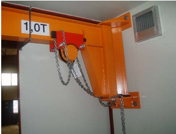
Swing crane inside the workshop
