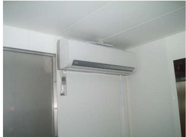
AC unit inside the control room.
