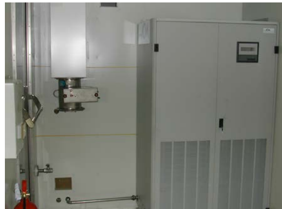
HVAC and VSD Cabinet
