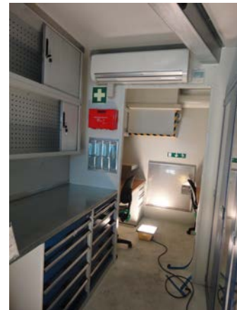
AC Unit above opening to office section
